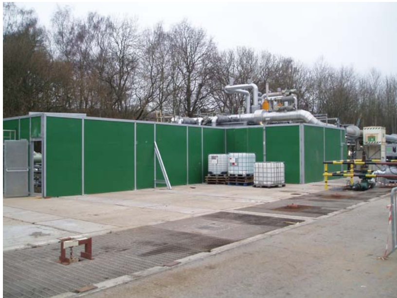
Photograph No 2 – Acoustic Fence on site at Humbly Grove Wellsite 'A', Hampshire.
