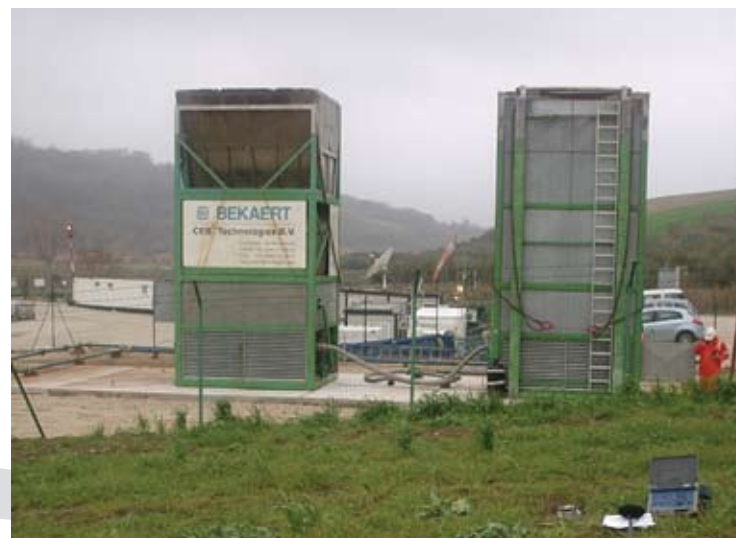
Clean enclosed burner - only one would be needed at Albury
